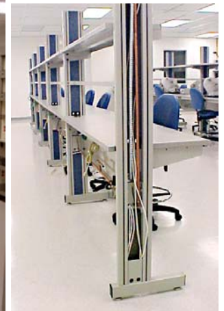
Vertical and horizontal utility run thru columns
