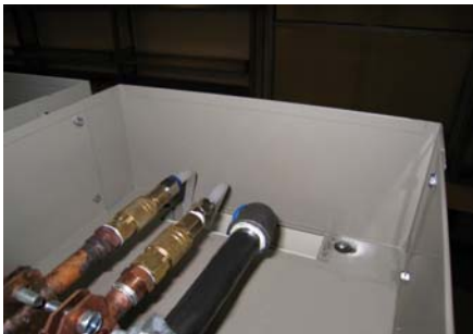
Overhead utility chase and tubing drops into top of column. Use of quick disconnects allows trim panels to be removed for modifications & additions to installed components.
