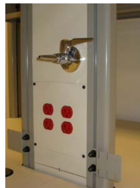
Gas valve and power outlets in wide column
